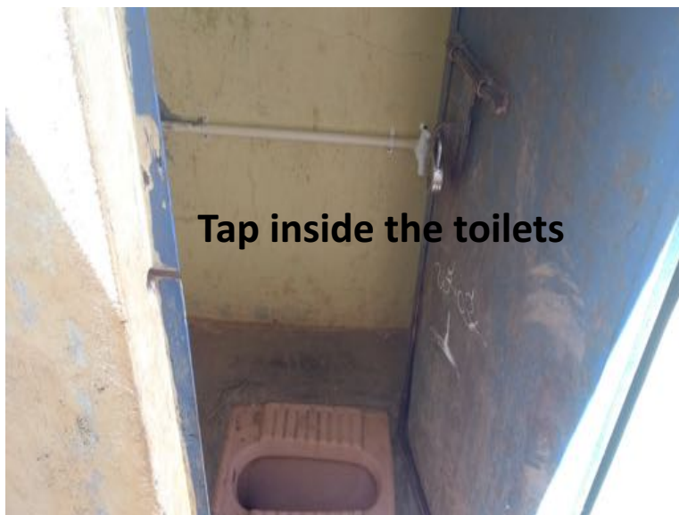
Plumbing connection to the toilets
