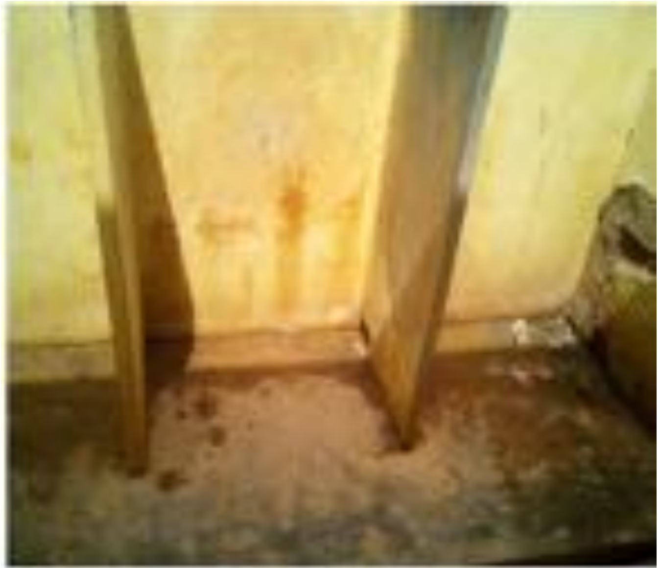
Urinals without appropriate drainage
