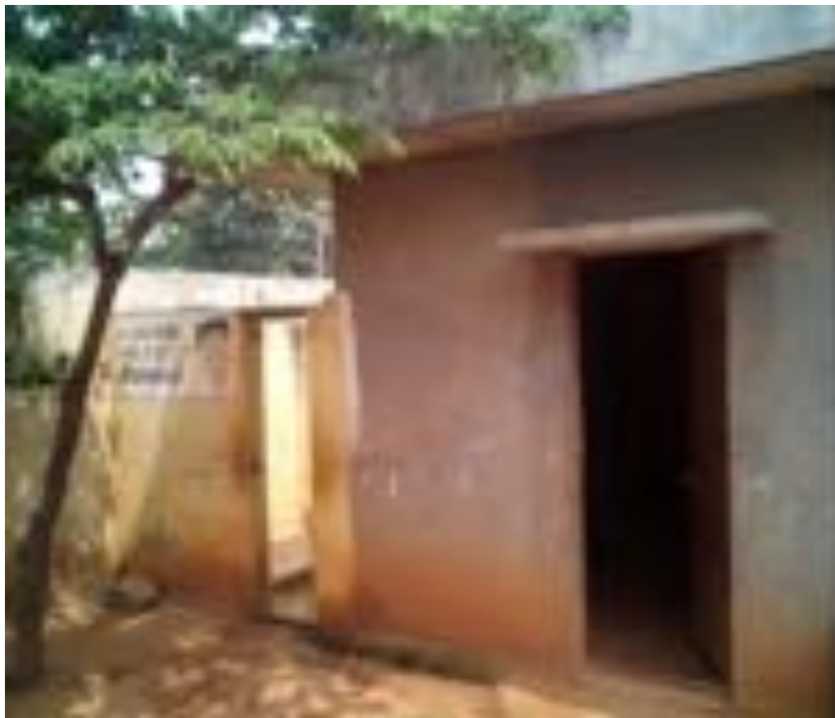
No plumbing to the toilets
