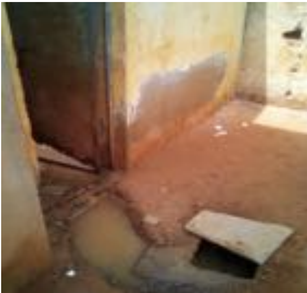
Water stagnation near toilet blocks, Broken toilet door
